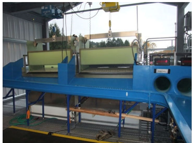
Stunning Grid and Sorting Area on top level. Fish come up from ground level via the "Pescalator."
